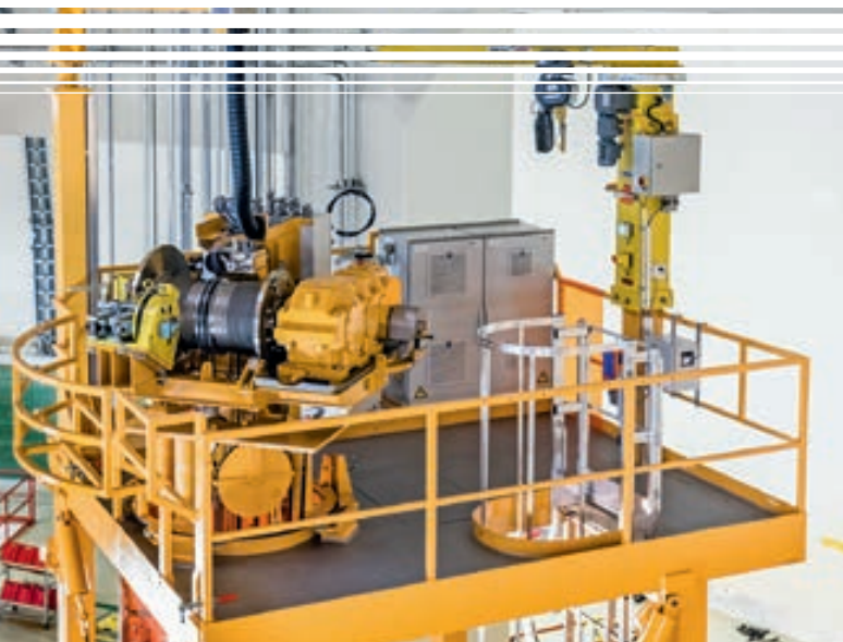
New installation of the lifting unit on the platform, with integrated access
