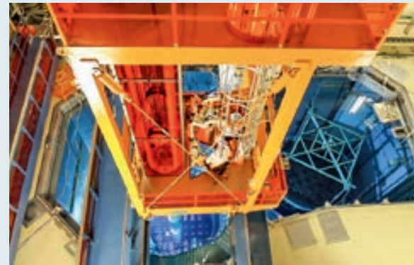
Refueling machine in operation above the reactor pool
