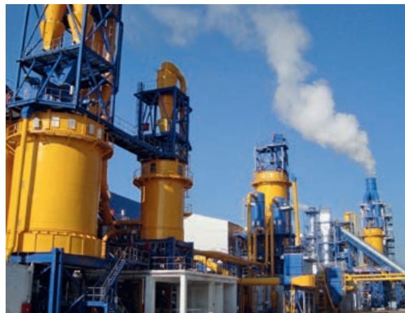
Silo discharge system
