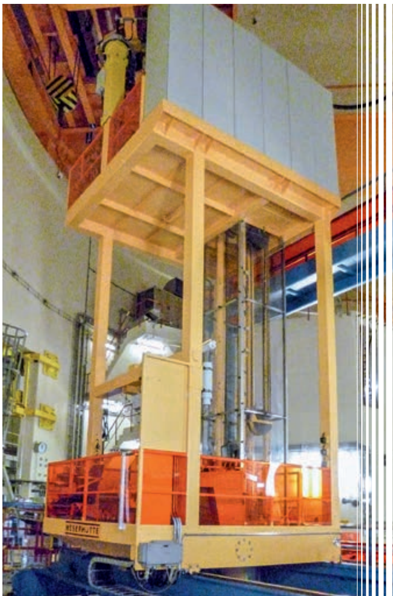
Refueling machine before refurbishment
