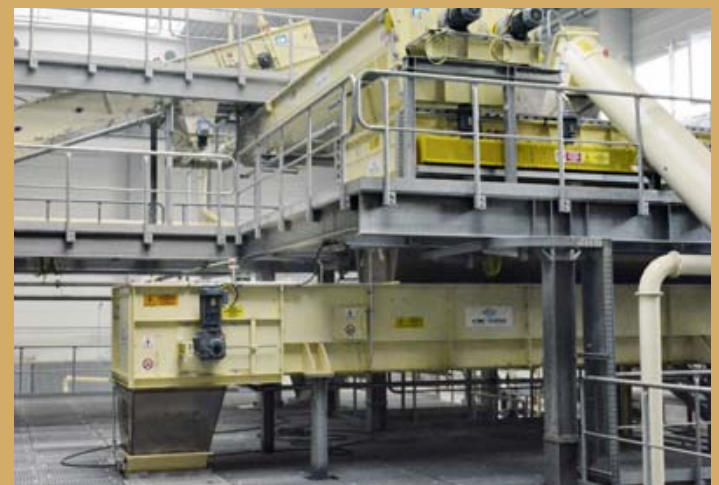
Disc screen above core layer mat-forming machines
