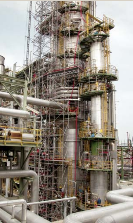
Testing and inspection work in the outside area of the TOTAL refinery
