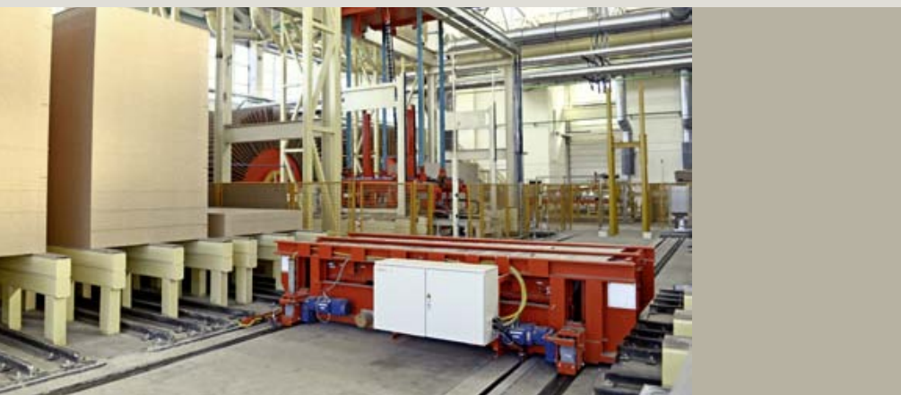
Cooling turner, intermediate storage and satellite vehicle
