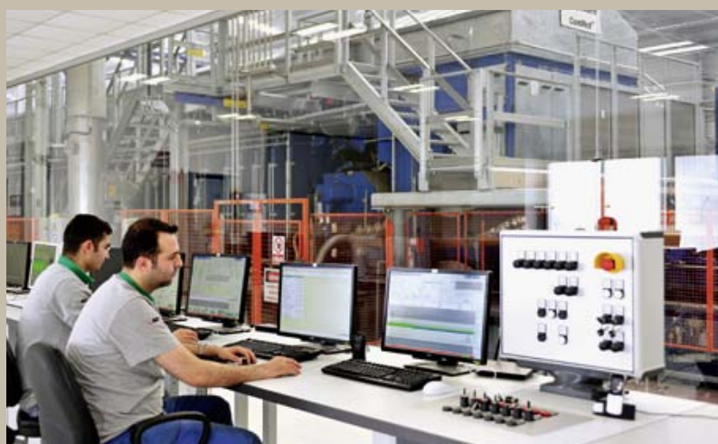
Control room of the plant
