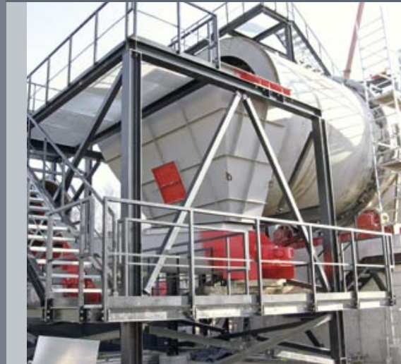
Installation in Gulbene: drum dryer discharge end, fan in the background
