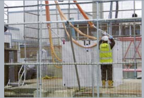
Mounting of the lifting device for the transport at a height of 5.20 m
