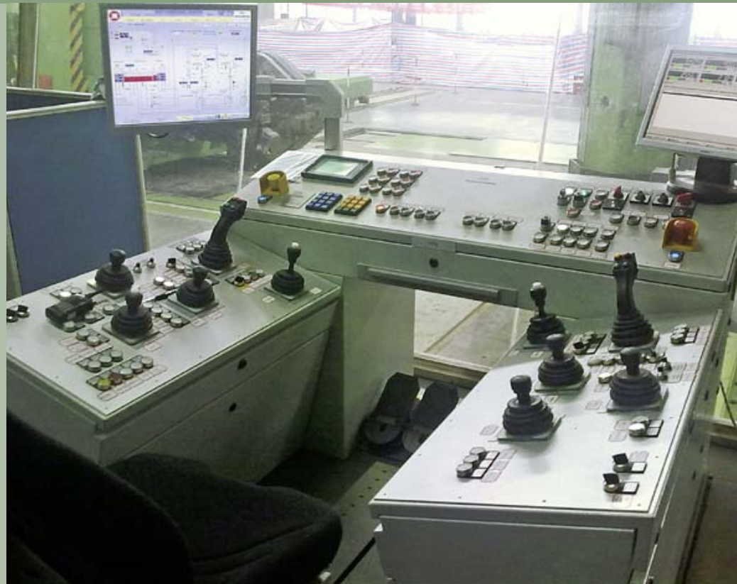
Press control after upgrade
